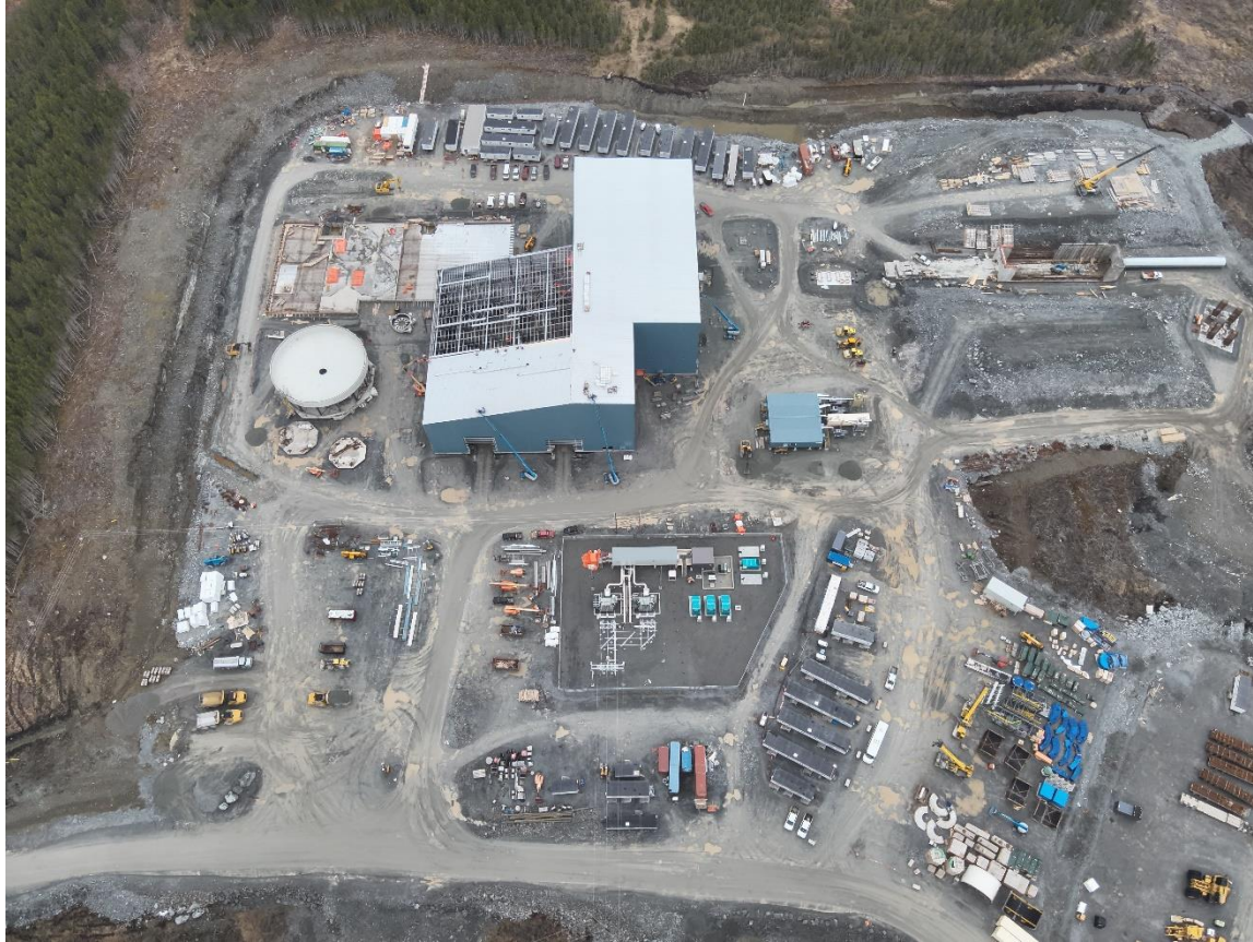
Process Plant East
