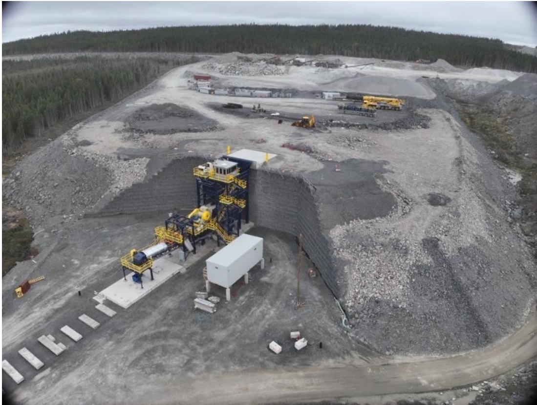
Primary Crusher Installation
